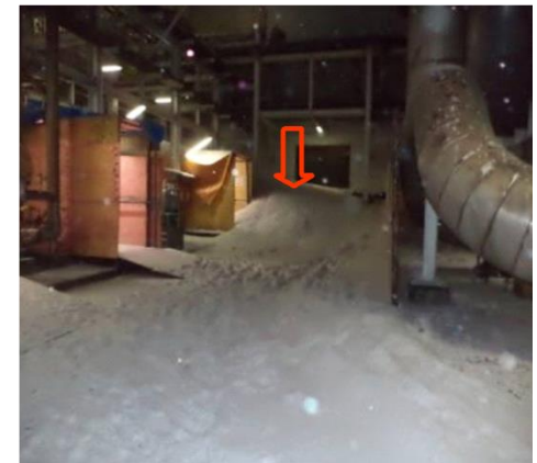
East side of coldbox after initial cleaning, immediately after release about 4 m of perlite was piled up here. Arrow indicate where the victim was found
